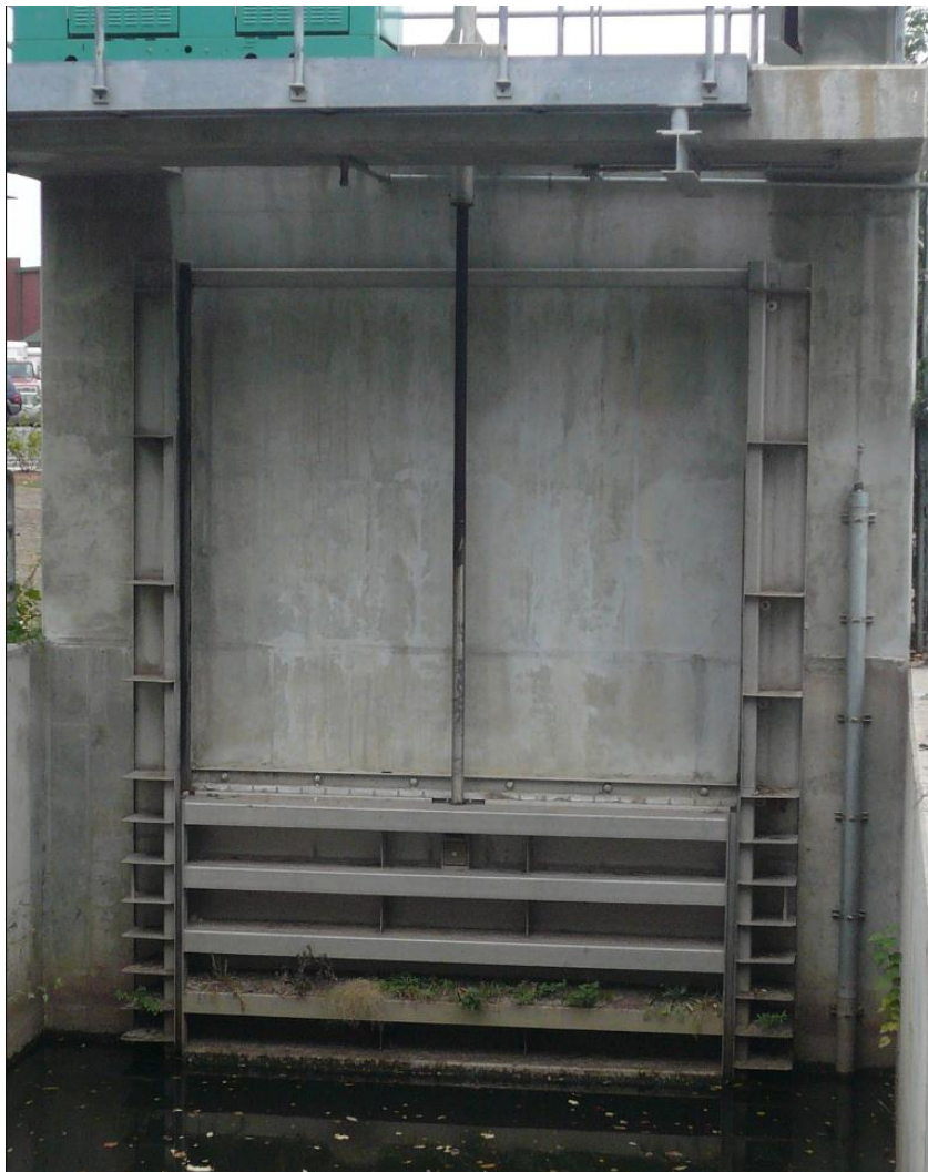
Figure 8: Photo of a sluice gate.
